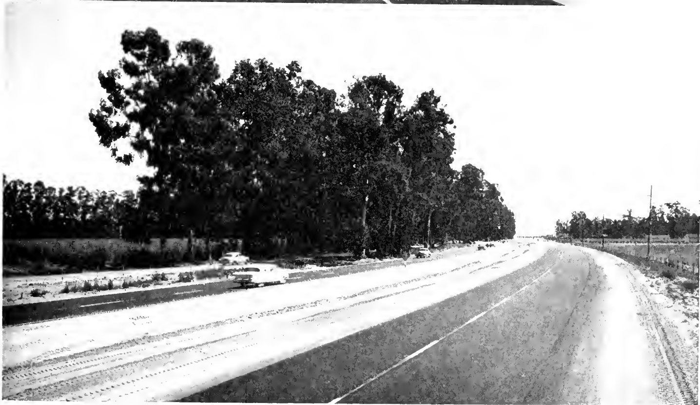
UPPER—View west in vicinity of Rose Road showing old highway right for use as north frontage road, taken just before completion of chain link fence and shoulder seal coat. LOWER—View toward east during latter stages of construction. Typical preservation of eucalyptus windbreak between new expressway and frontage road. Eastbound lanes at this point had not yet been put in operation.
